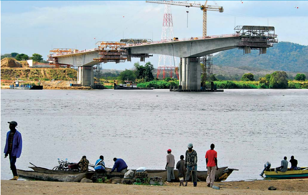
Construction of a new bridge over the Zambezi river near Caia. Improved physical infrastructure is important to digital inclusion but so are the skills to make use of technology and the ability to pay for it.
